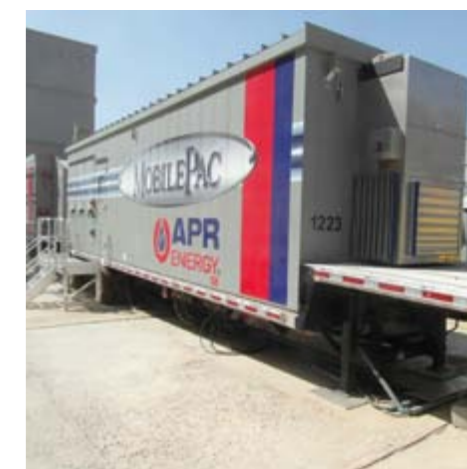
□ APR's electrical mobile generator
