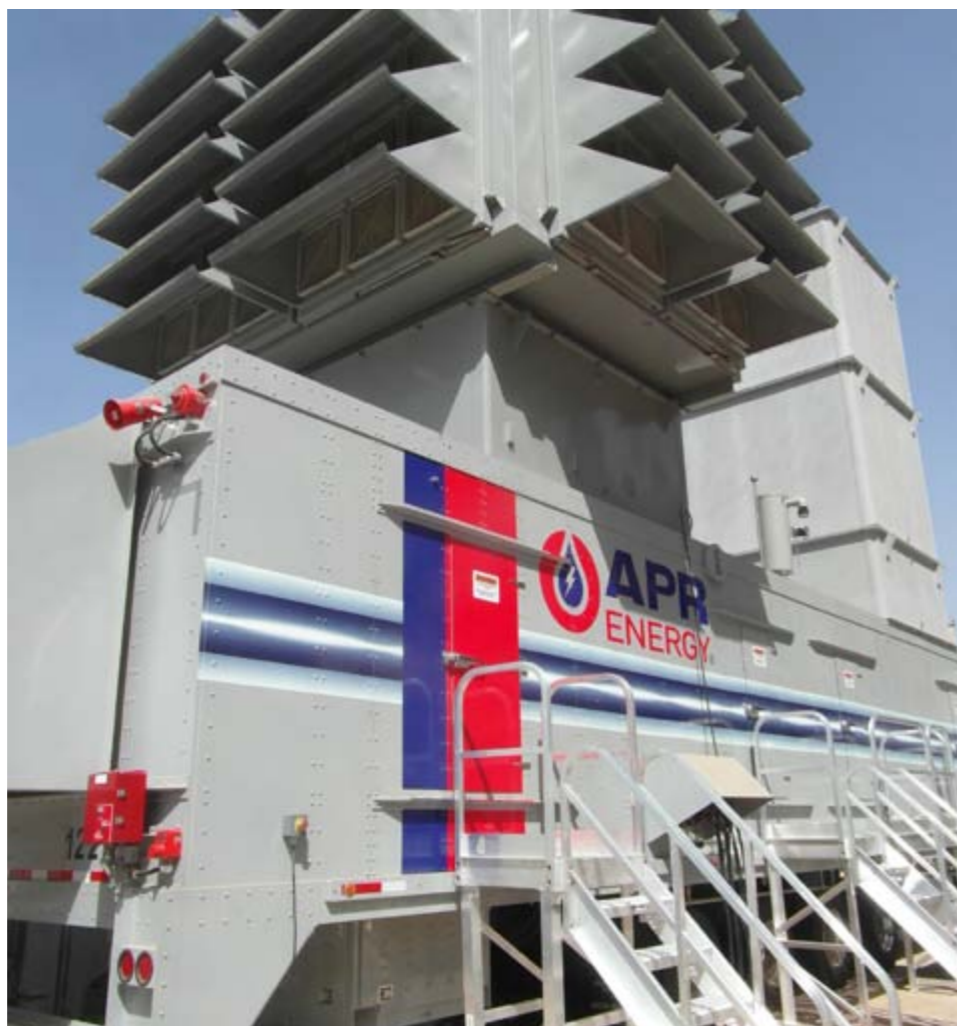
□ APR's electrical mobile generator
